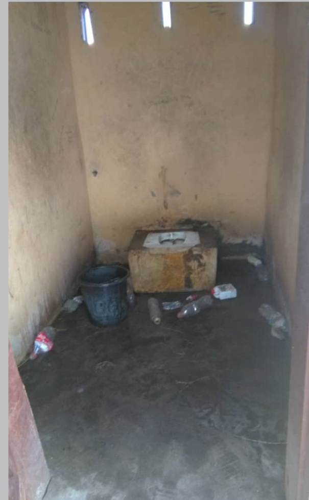
Another toilet at Community Junior High School Akodo –Orofun, Lekki Town, Lagos
